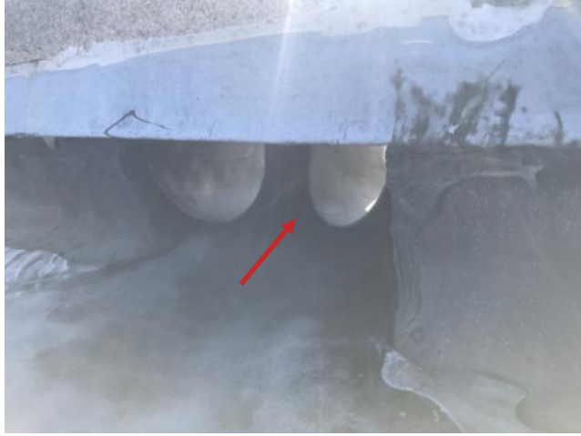
Drain Point Flashings Wide Open
