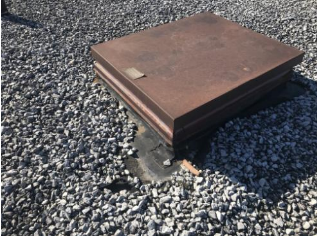
Curb Flashings Old But Holding
