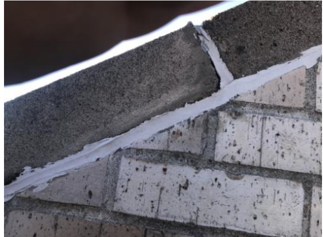
Cap Stone Joints Starting To Open
