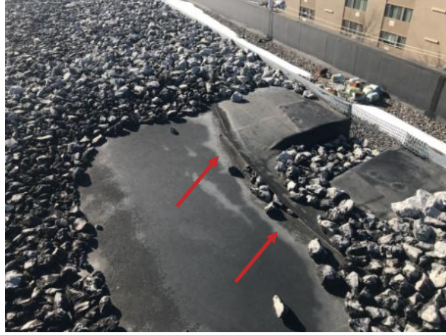
Lifting Seam At Drain Point
