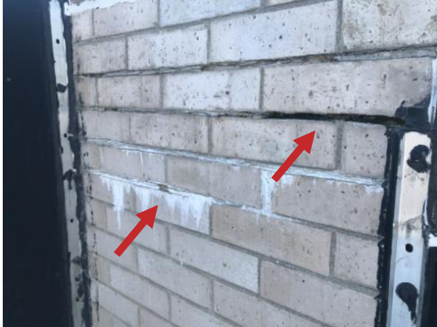
Open Joint Causing Efflorescence
