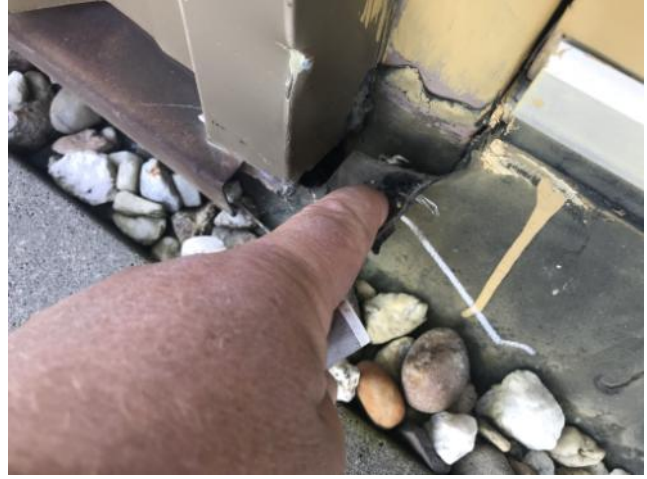
Various Holes & Openings Noted
