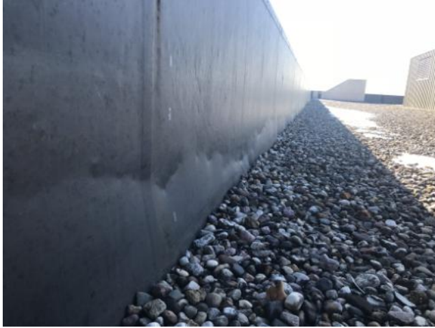
Minor To Moderate Pulling (Common)
