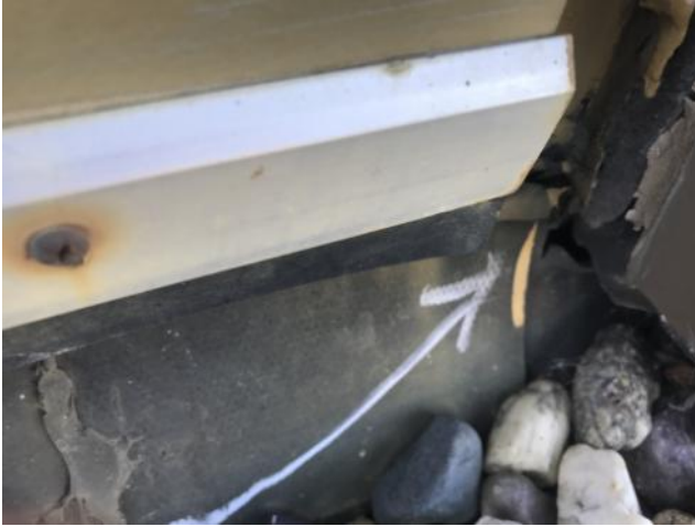
Various Holes & Openings Noted
