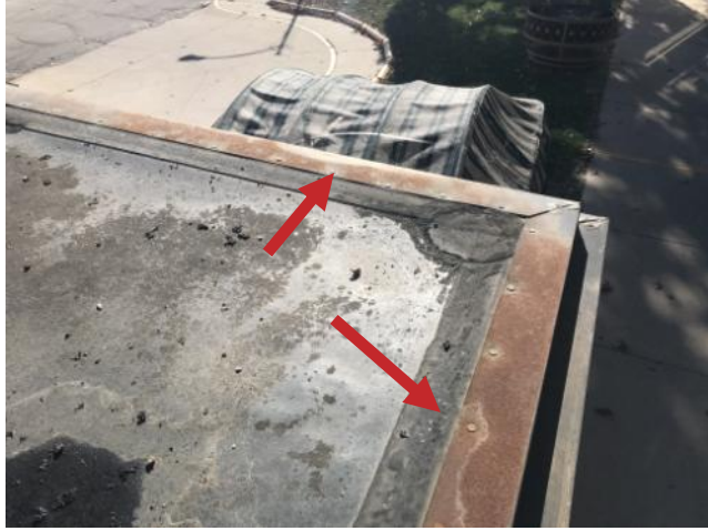
Flashing Is Supposed To Be Over Nails
